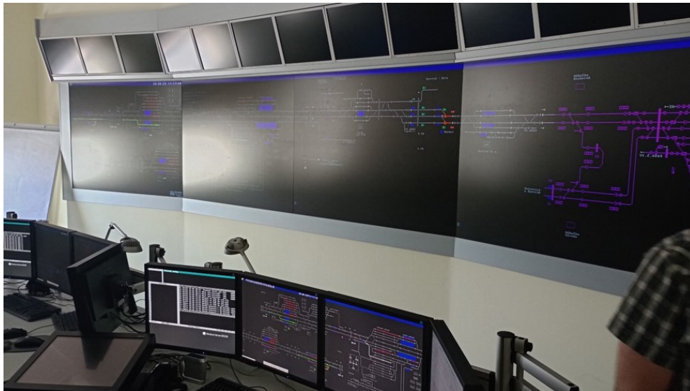
Fig. 1. Sample local control center
