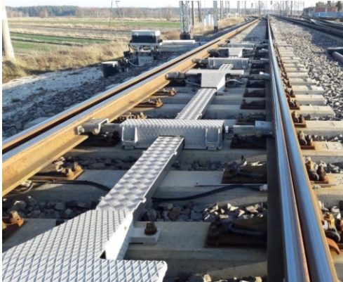
Fig. 4. Switch area [Source: Authors library]
